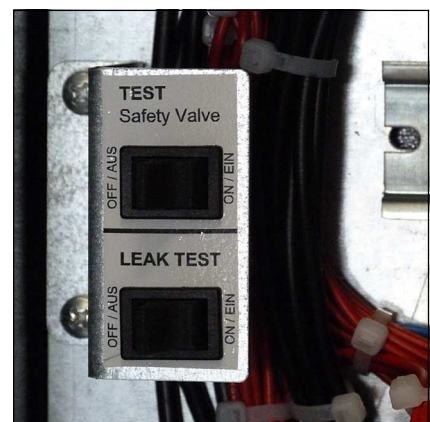
Leak test switch (down)
