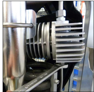
Fig. 1 - Loosen pipe connections
