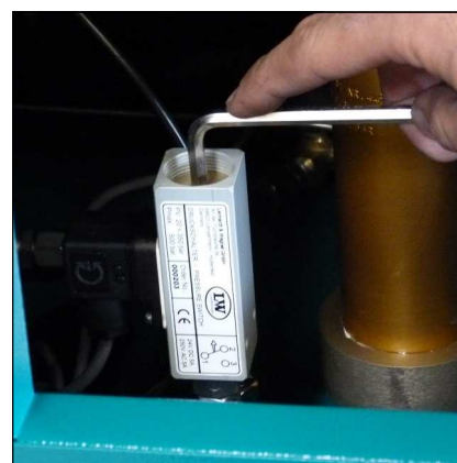
Final pressure switch
