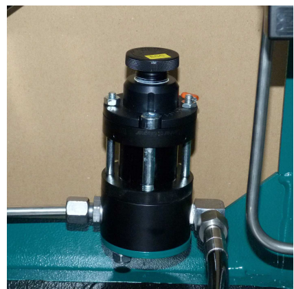
Safety valve 3rd stage
