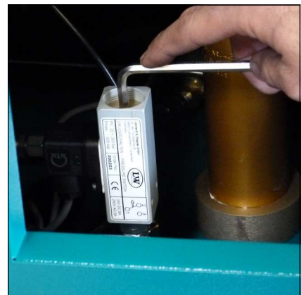
Final pressure switch
