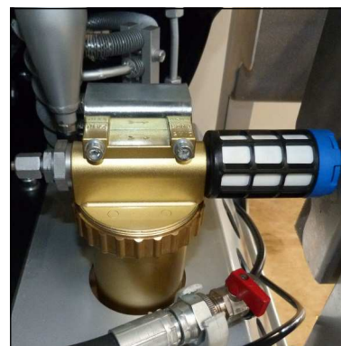
Oil / water separators final stage
