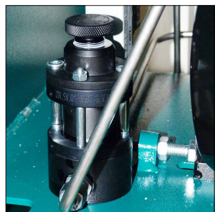
Safety valve 3rd stage
