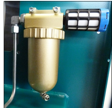
Oil / water separators final stage
